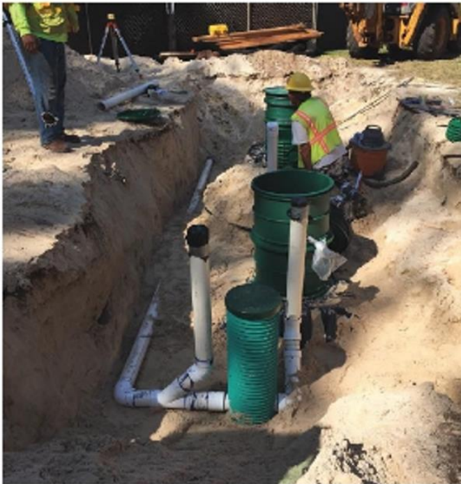
Construction of one of the treatment trains. It is a view of the risers coming up from the tank openings to grade level for maintenance access.
