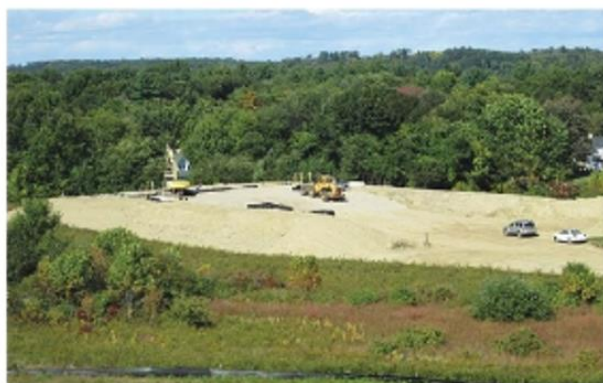
The system was designed in an elevated mound configuration, due to separation to seasonal high-water table requirements for new construction.
